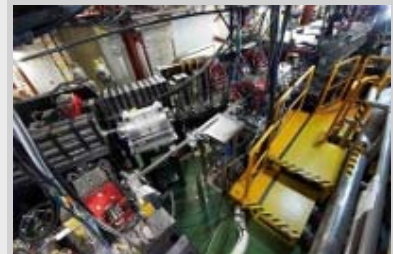
Two units of the strip-line kickers installed at the ATF damping ring.
