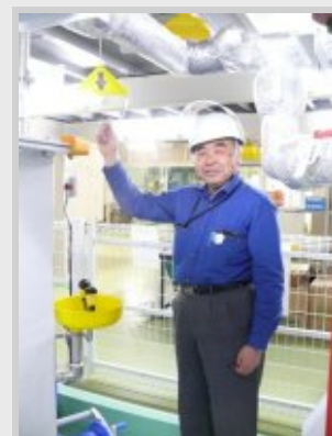
Funahashi showing the emergency shower system.
