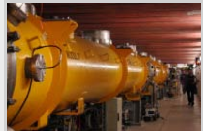
Six modules installed in FLASH at DESY have 48 nine-cell cavities operating between 20 and 25 MV/m. The nine-cell TESLA cavities inside the module were fabricated from RRR=300 niobium and prepared by advanced methods of electropolishing and baking.
