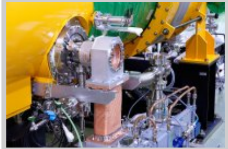
Input coupler connected to a cavity (baseline design) at STF cryomodule A. (Photo KEK)
