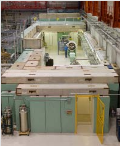
Fermilab will use Recovery Act funds to expand its superconducting radio frequency test facility and make cryomodules to construct a prototype accelerator.
