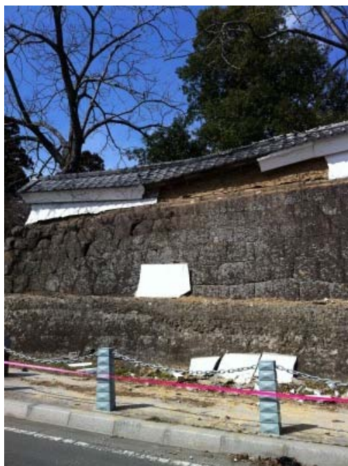
Damage to the walls of Sendai castle after 11 March earthquake.
