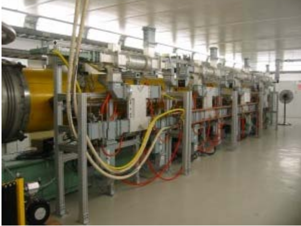
CM1 with its recently installed RF distribution system ready for testing. Image: Jerry Leibfritz
