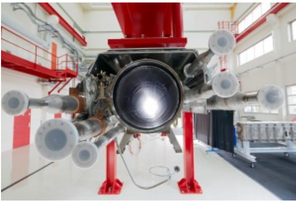
Cryomodule production for the European XFEL in CEA Saclay, France. Image: DESY
